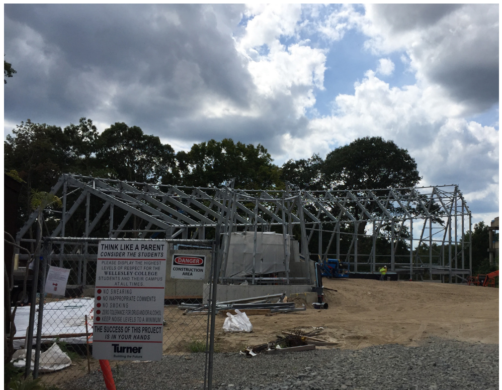
The steel frame of the new greenhouse, 202 beams, 62 columns and 31 bracings, is now complete!
